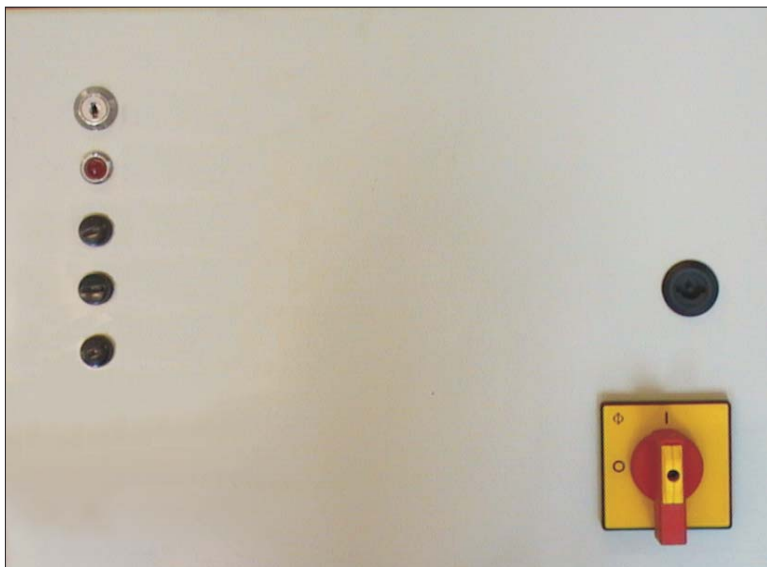
Main Control Panel
