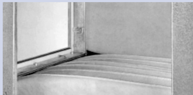
Ducted bag filter with standard cell frames
